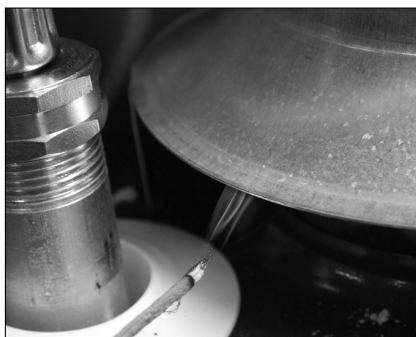
Figure 33: Test the air supply and vent to make sure the water heater has adequate air and is venting properly.
