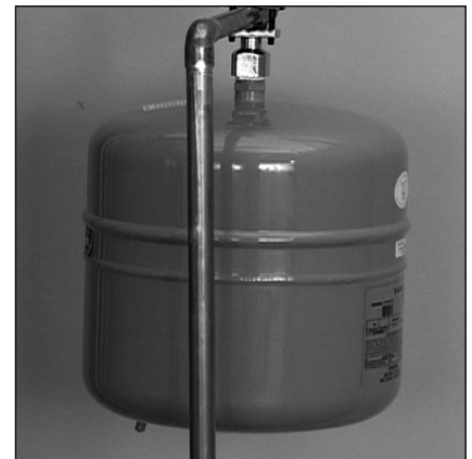
Figure 23: The Thermal Expansion Tank should be pressurized with air, using a hand pump, to match the home's incoming water pressure.
