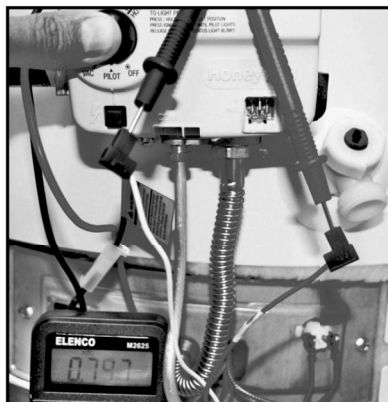
USE A MULTIMETER TO CHECK THE OUTPUT OF THE THERMOPILE (MEASURED IN MILLIVOLTS). SHOWN ABOVE - MULTIMETER PROBES ARE INSERTED INTO THE THERMOPILE PLUGS. THESE PLUGS WERE REMOVED FROM THE RECEPTACLE AT THE BOTTOM, RIGHT-HAND CORNER OF THE GAS CONTROL VALVE/ THERMOSTAT.
