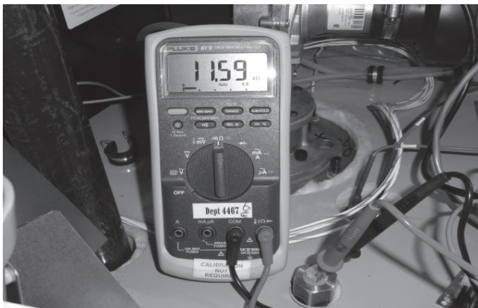
Temperature Sensor Test
