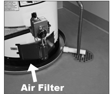
Figure 24 - Filter attached to water heater.
