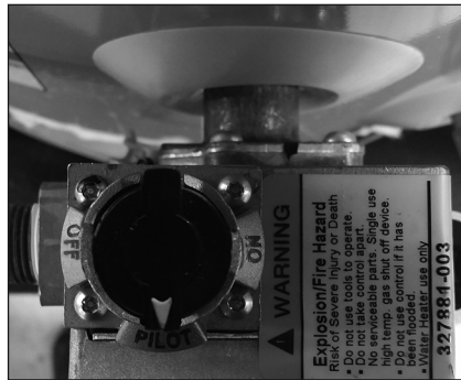
Figure 34 - Gas control/valve top view.
