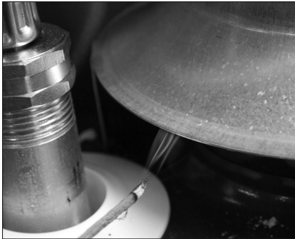
Figure 36 - Test the air supply and vent to make sure the water heater has adequate air and is venting properly.
