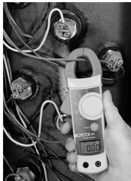
Figure 18. Heating Element Amperage Test
