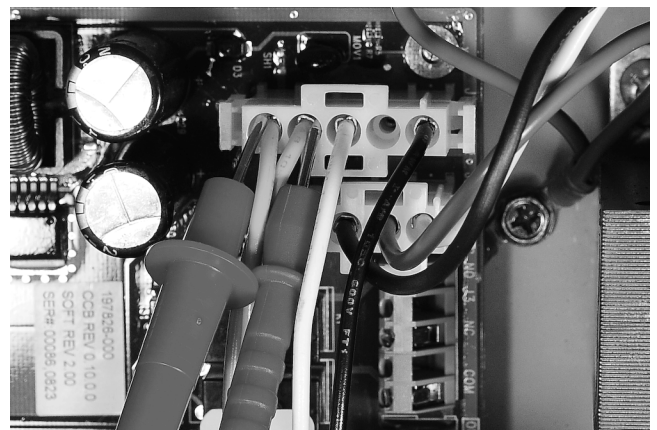
Figure 35. 24 VAC Transformer Secondary Winding Voltage Test
