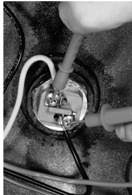
Figure 19. Element Voltage Test
