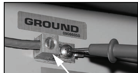
Water Heater Ground Connection
