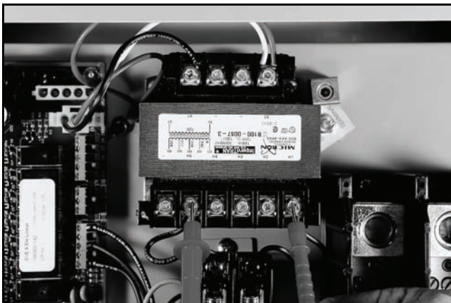
Primary Winding Voltage Test
